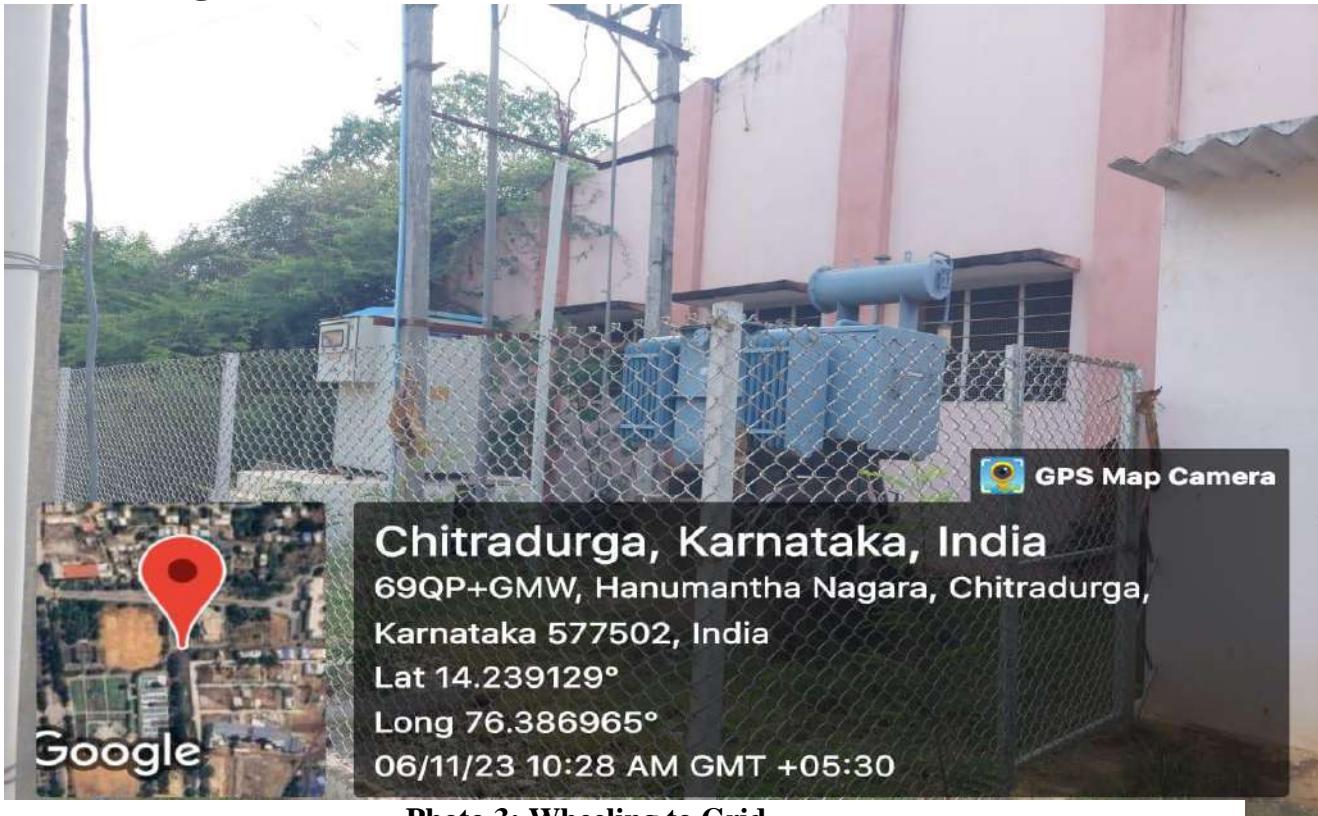
Photo 3: Wheeling to Grid
