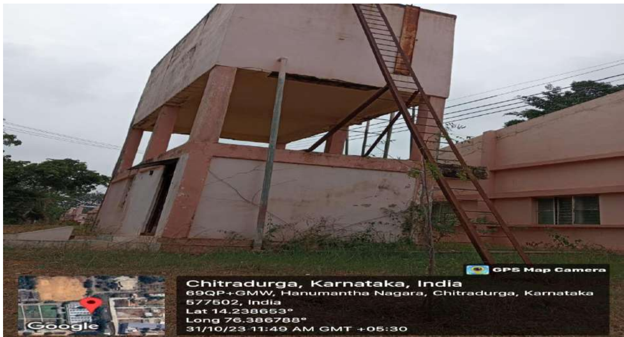
Photo 20: Over Head tank
