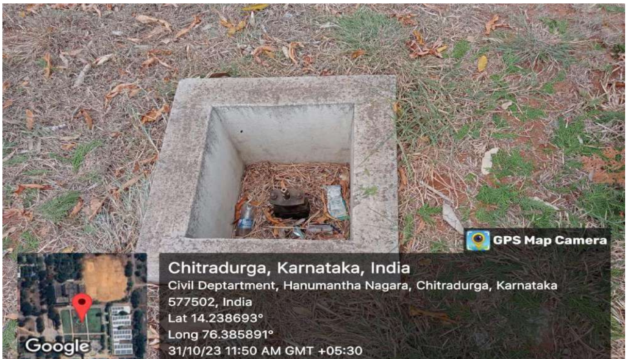
Photo 12: Valves provided for Supply of water
