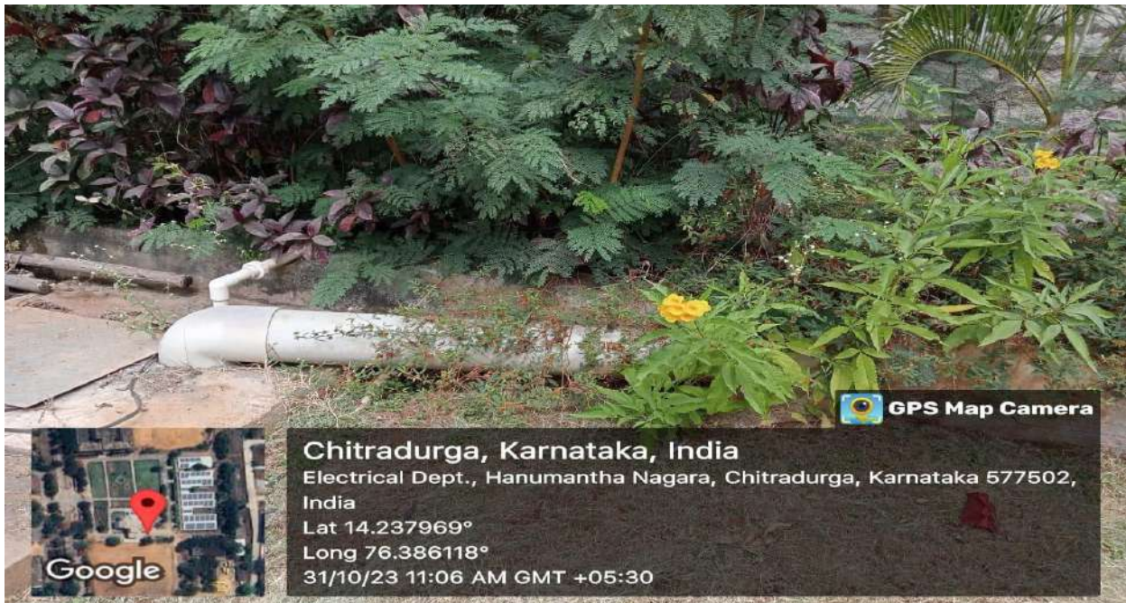
Photo 17: Rain Harvesting Sump tank at administrative building
