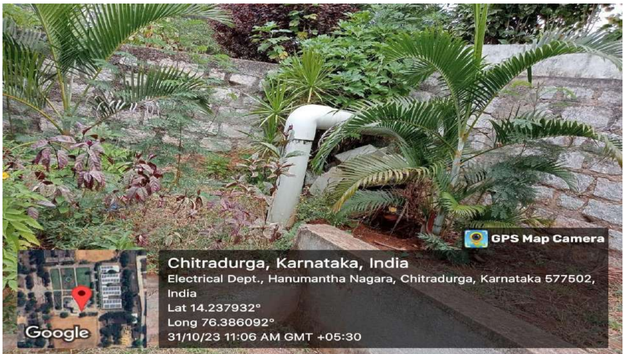
Photo 18: Rain Harvesting Sump tank at administrative building
