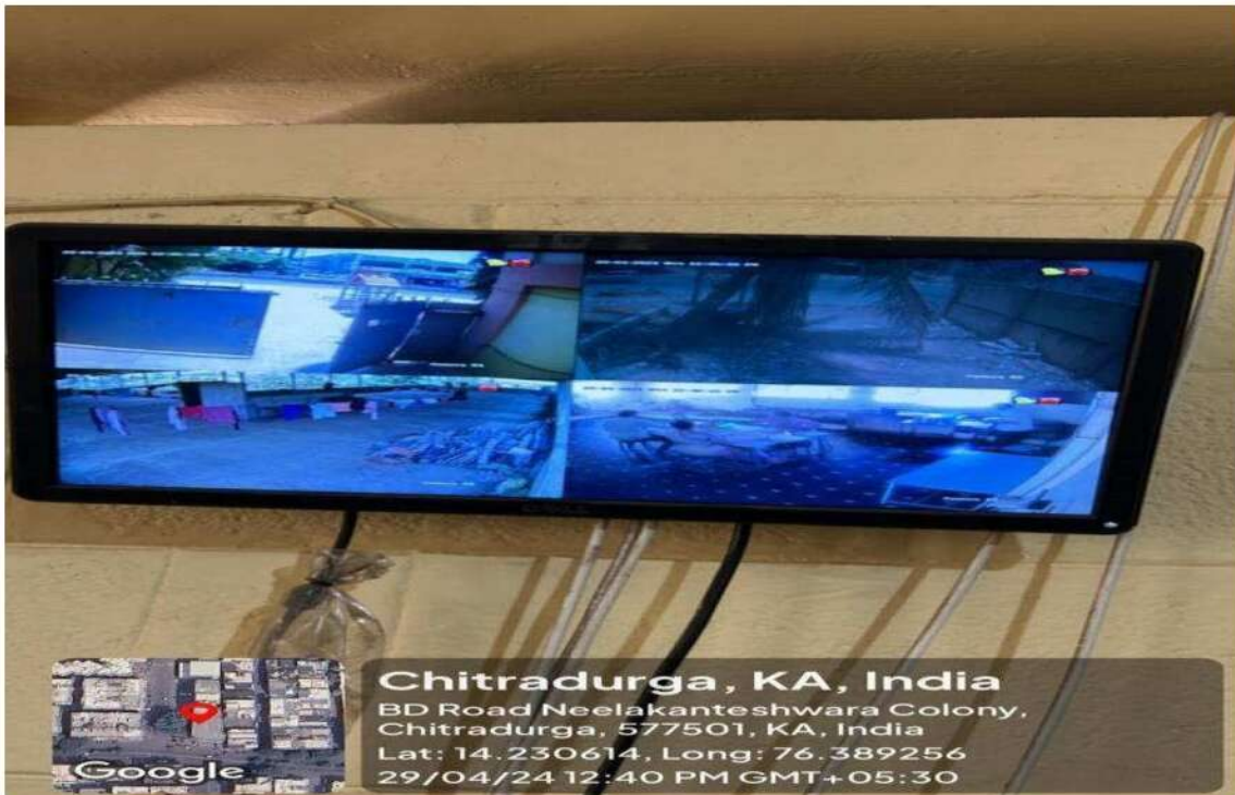
Photo 16: CC TV monitoring at Ladies Hostel
